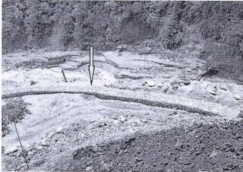
Figure- 1: Erected Gabion wall surrounding the periphery of muck disposal site near T4
