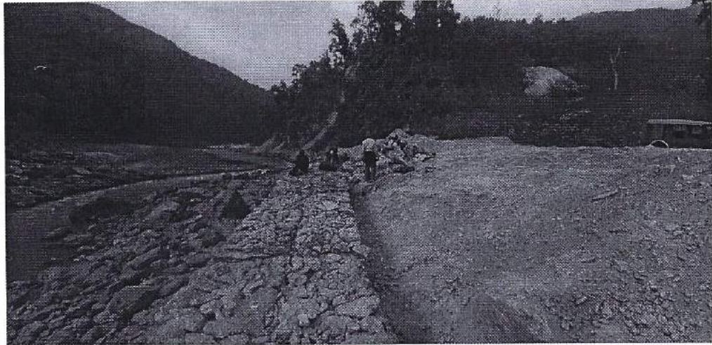
Figure- 2: Erection of Gabion wall surrounding the periphery of muck disposal site along Teesta River
