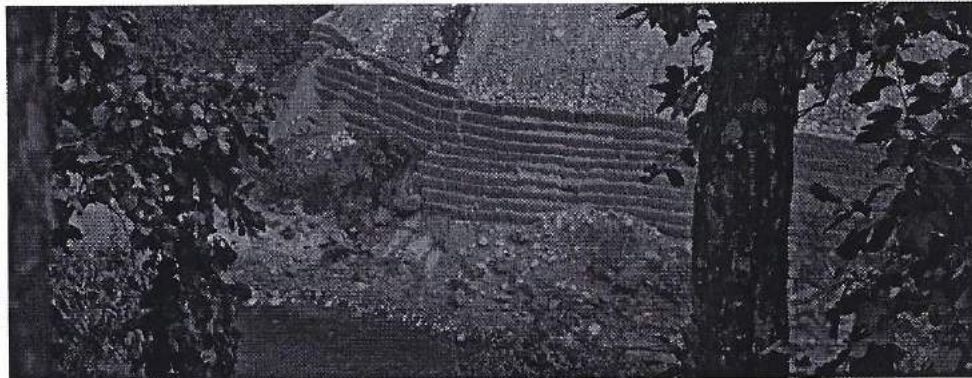
Figure- 3: Step-wise erection of Gabion wall surrounding the periphery of muck disposal site to provide the stability
