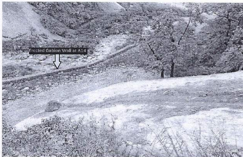
Figure- 4: Erected Gabion wall surrounding the periphery of muck disposal site at A14 for muck generating from T9 & T10
