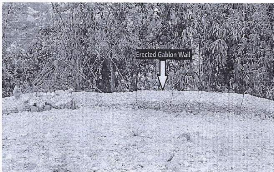
Figure- 2: Erected Gabion wall surrounding the periphery of muck disposal site near T5
