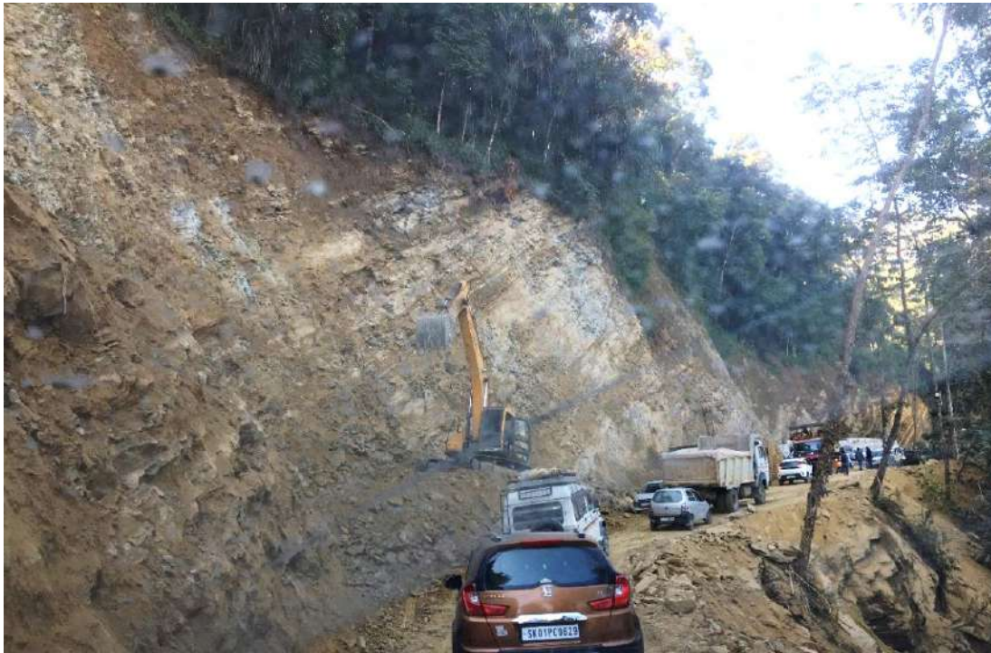
Figure 17: Mountain road construction is a challenging task and conventional wildlife over passes are not feasible
