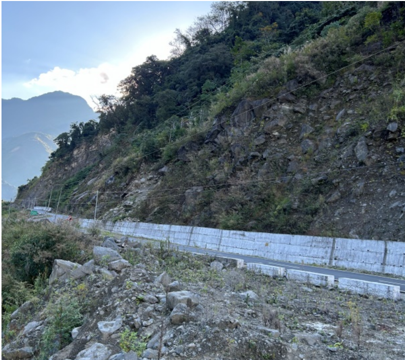
Fig. 8 View showing the debris deposit noted near the Penstock Alignment
