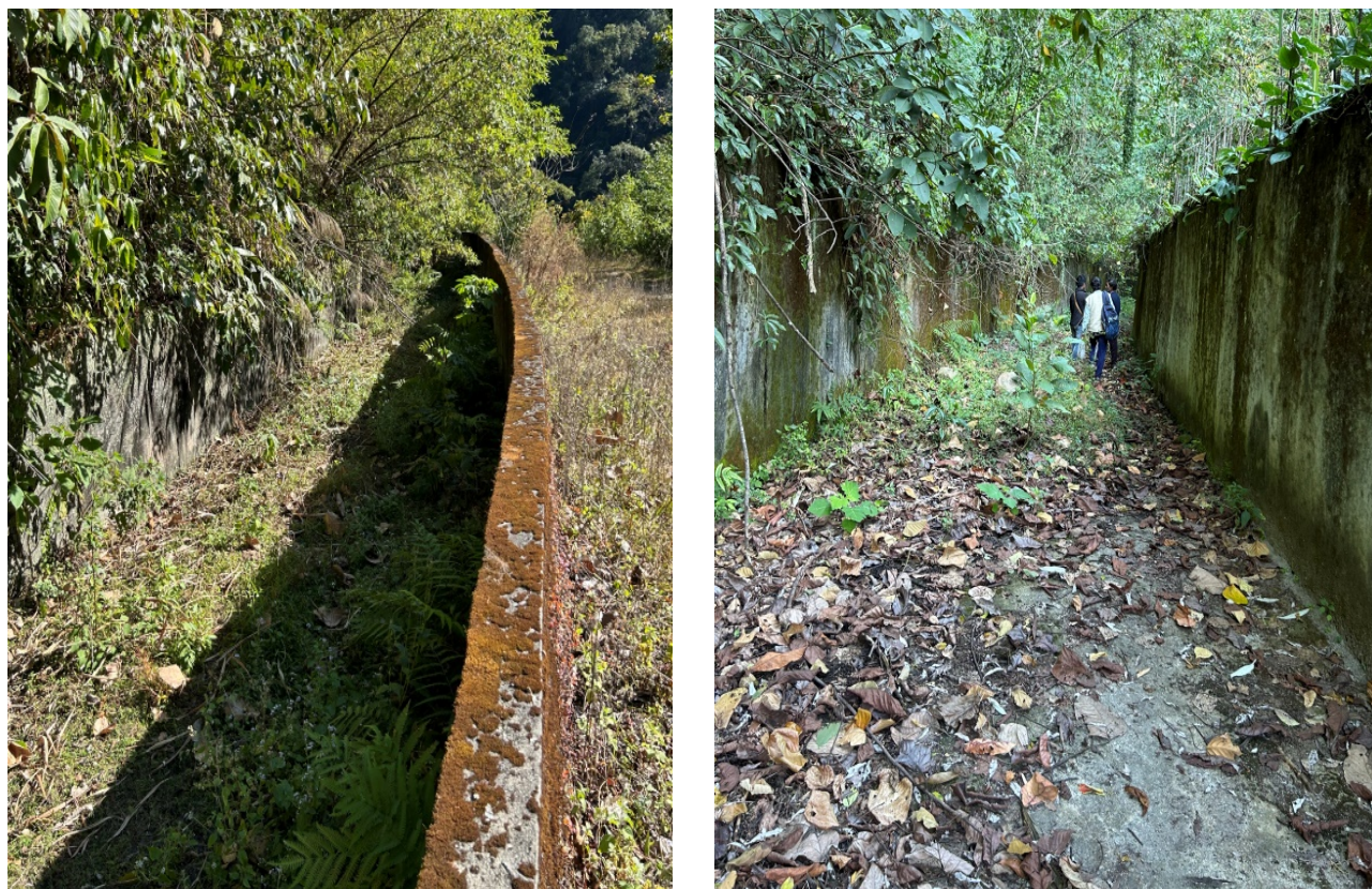
Fig. 16 A view showing the existing channel filled with sand/silt
