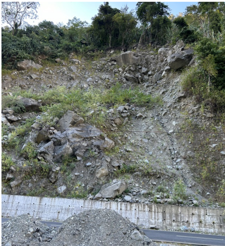
Fig. 9 A View of landslide beside the Anchor/Saddle block for penstock
