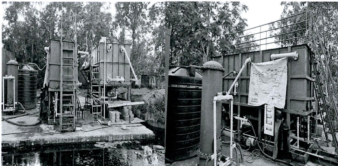
Fig. 1: Effluent Treatment Plant (ETP) at rig site
