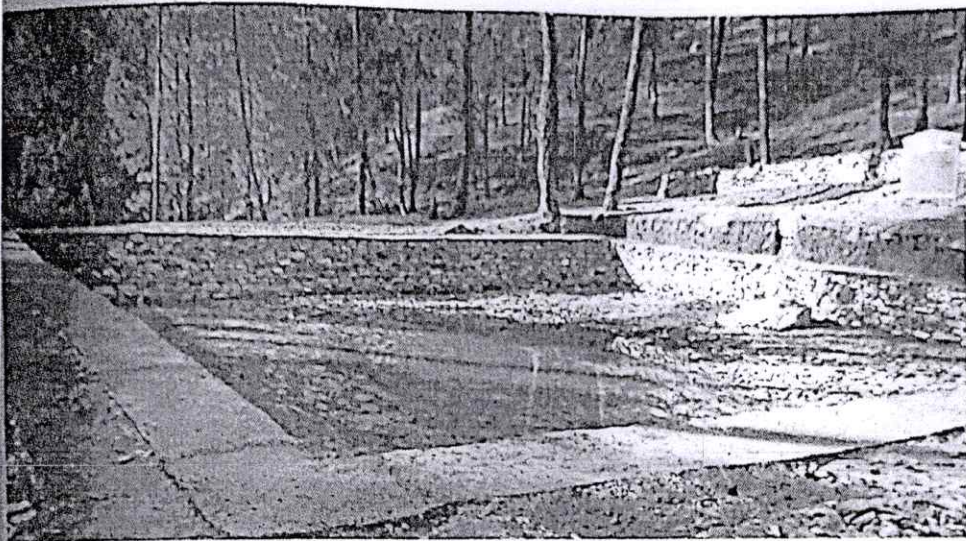
Water Harvesting Tank
