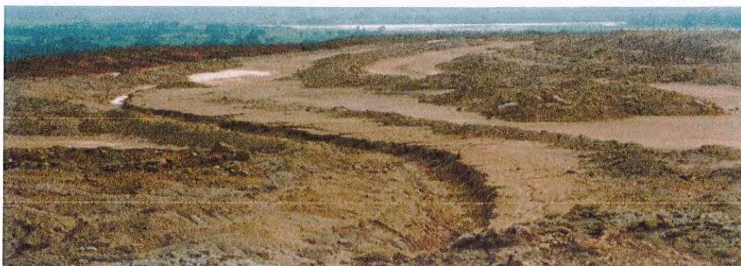
OB Management – Making garland drain to bring down run off in controlled manner
