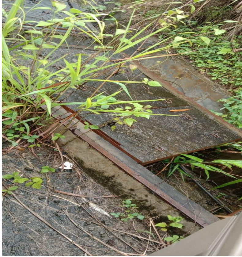
RCC Drain and Trench accommodating cables, etc
