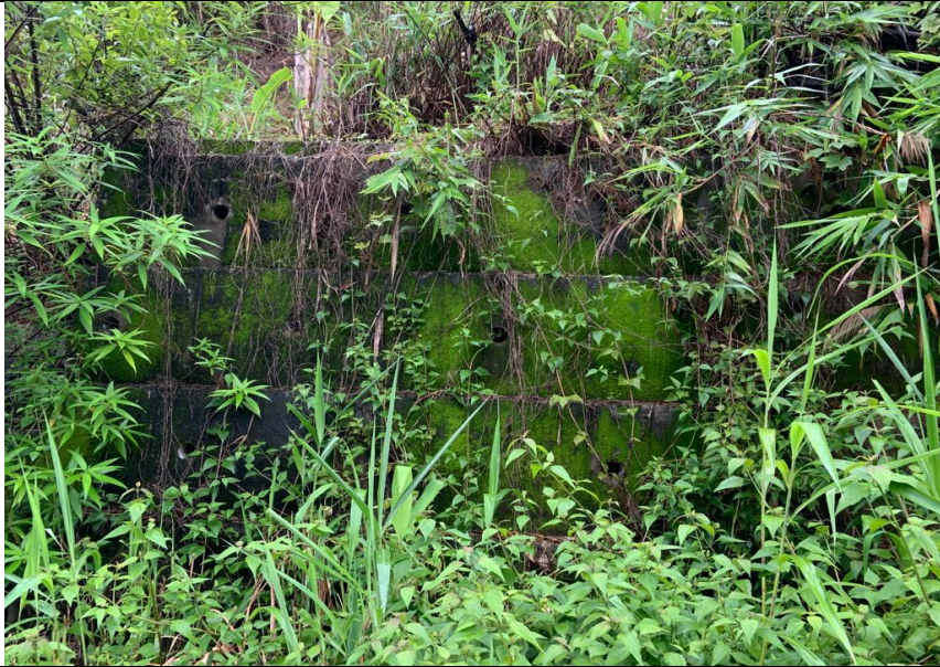
RCC Boundary Wall covered with moss
