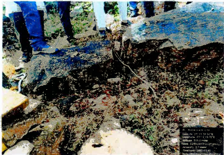
Field Photograph 04: Location of Powerhouse with VPS
