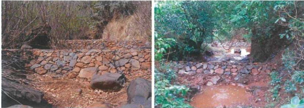
Fig 6.7: Loose boulder structure
