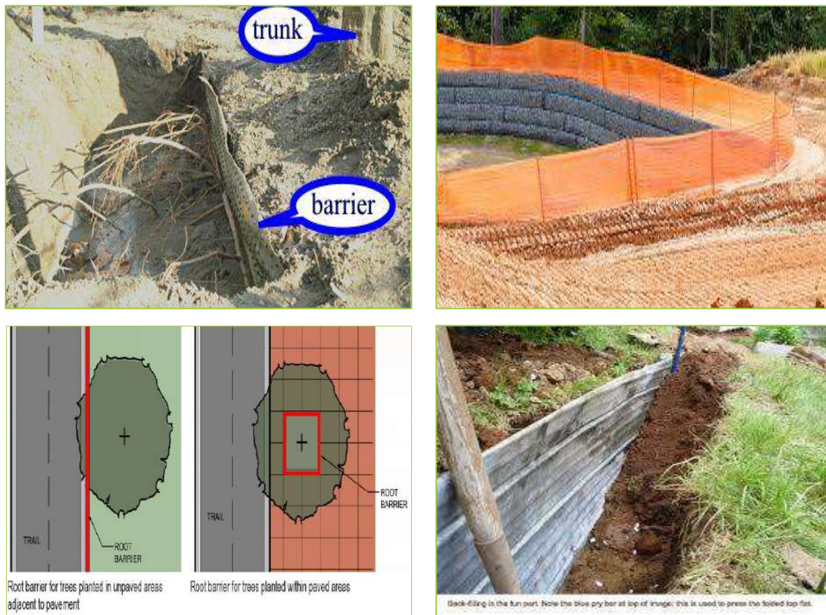
Figure 6: Provision of Barriers
