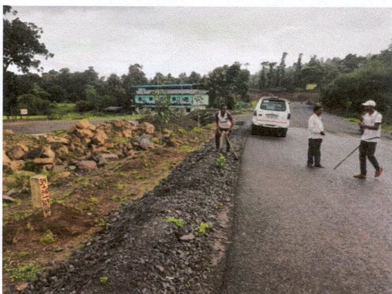
Ch. 34+840 (Left) pole 519
