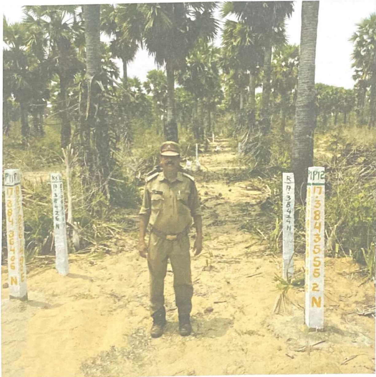
Erection of Concrete Pillars 4 feet high cement concrete pillars duly numbered at an interval of 20 meters in Gudivada Village of S.Rayavaram Mandal by M/s K.S.R.Prince Hatcheries
