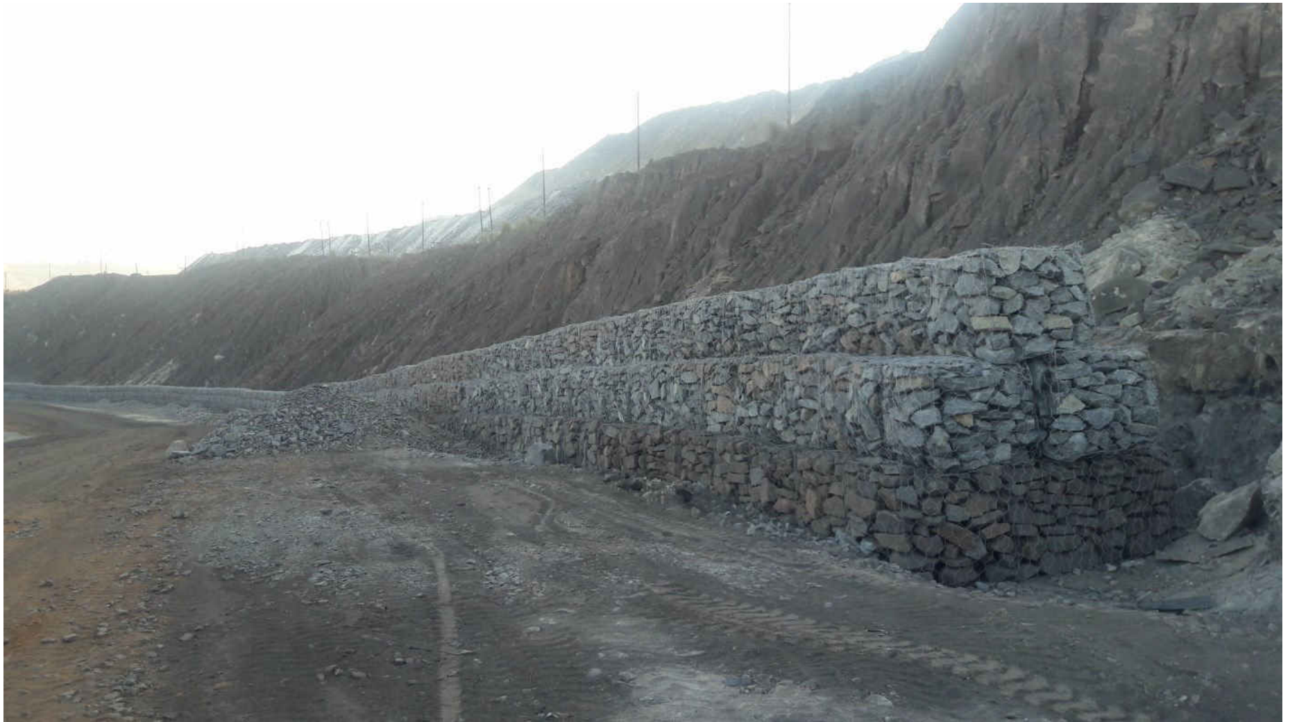
Gabion wall (3m X 3m for 0.5 Km ) along the toe wall of approach road
