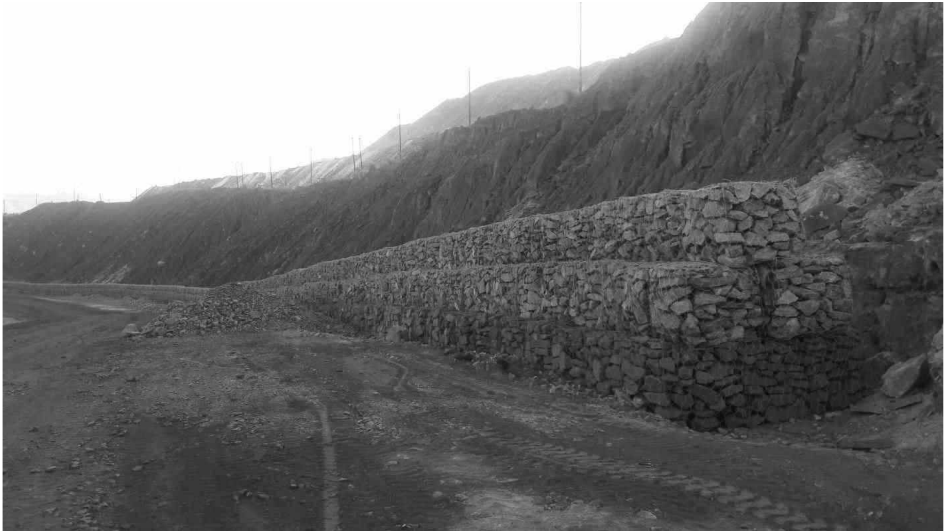
Gabion wall (3m X 3m for 0.5 Km ) along the toe wall of approach road
