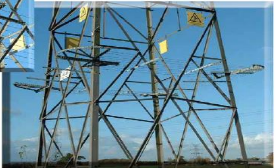
132kV TOWER ACD's
