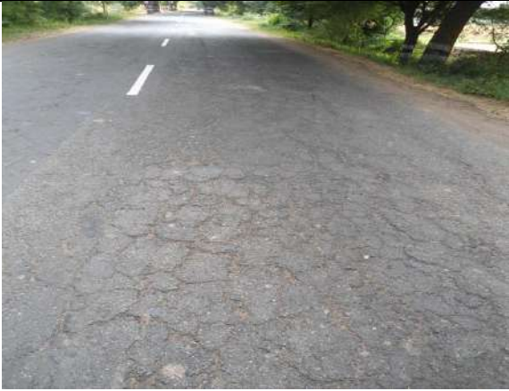
Severely Distressed at Km 6+000
