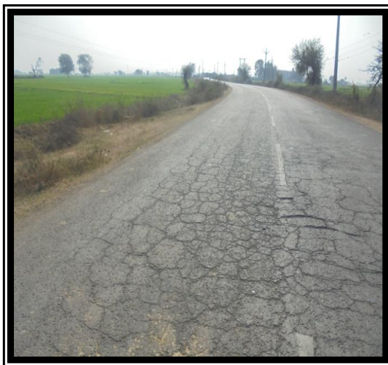
Photo-; Pavement Condition at Rural Section
