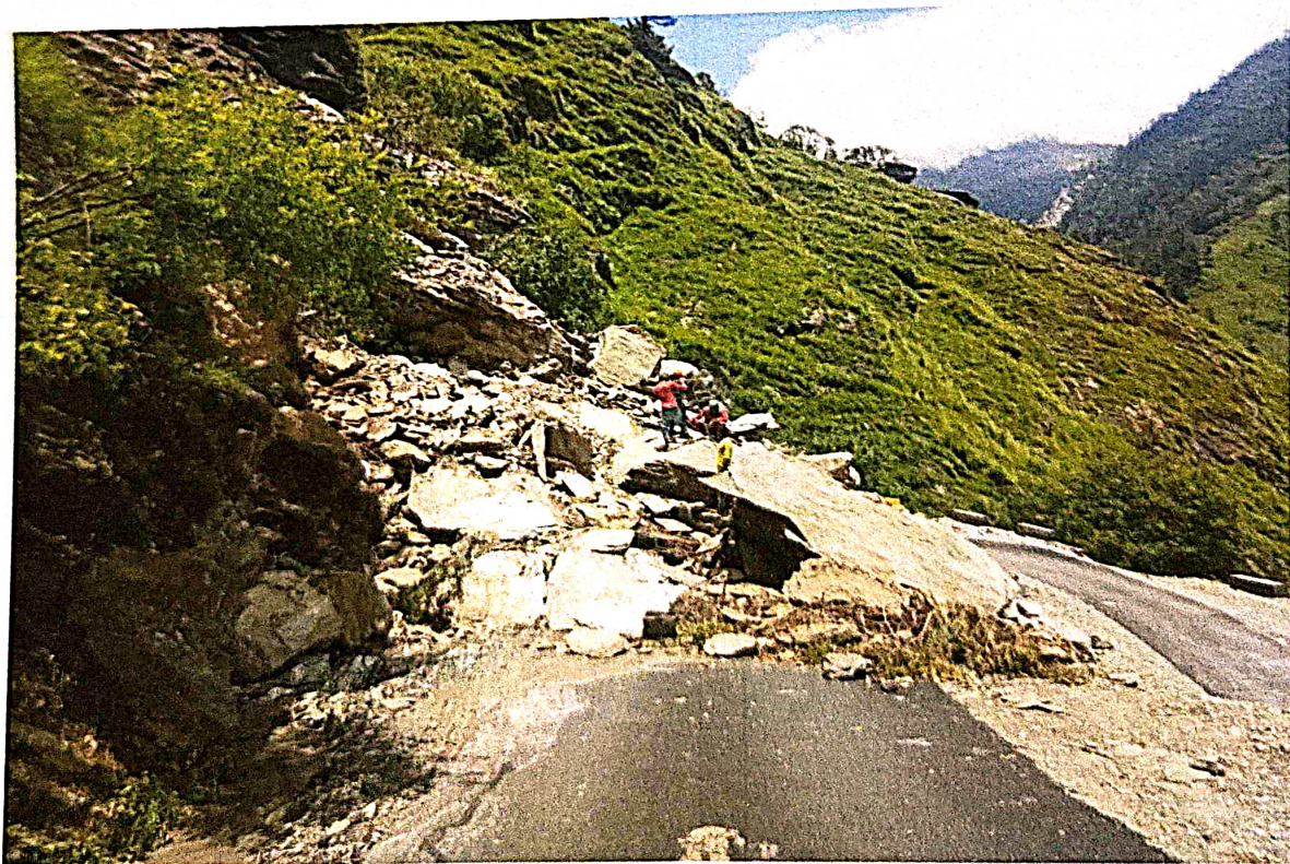
Slip and sliding Due to Monsoon
