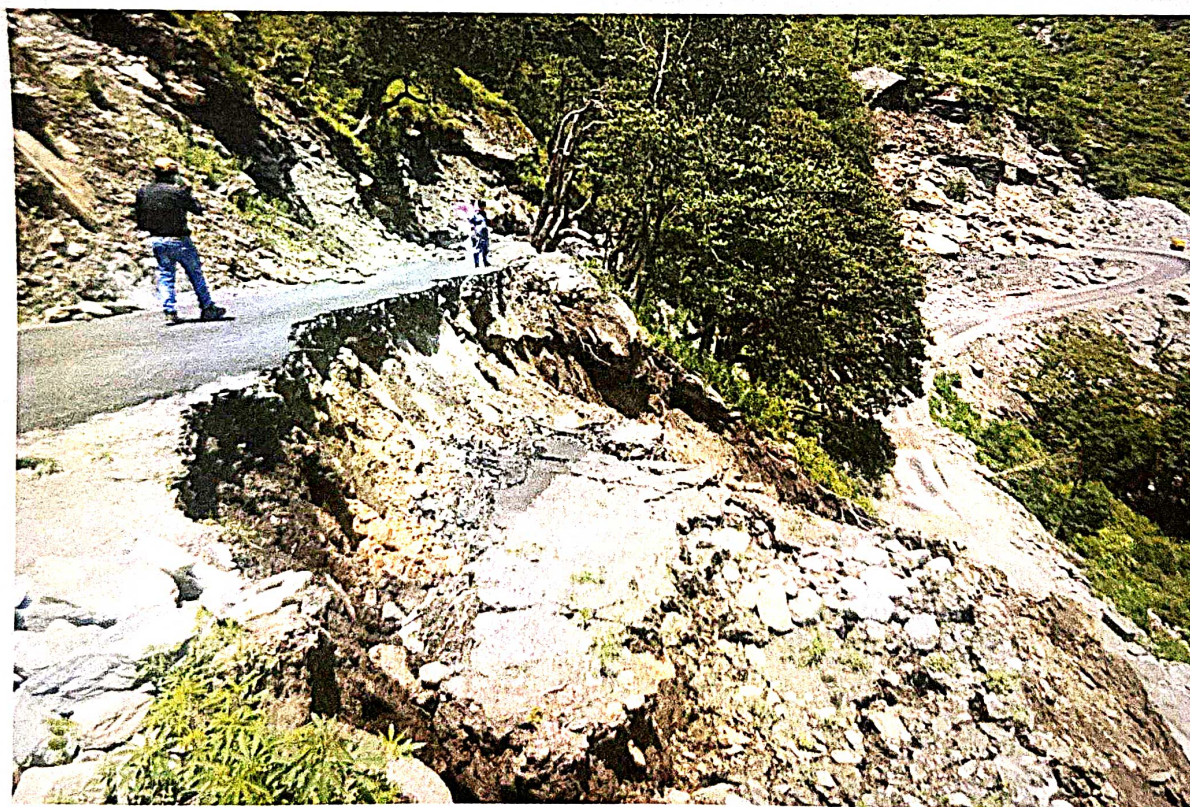
Slip and sliding Due to Monsoon
