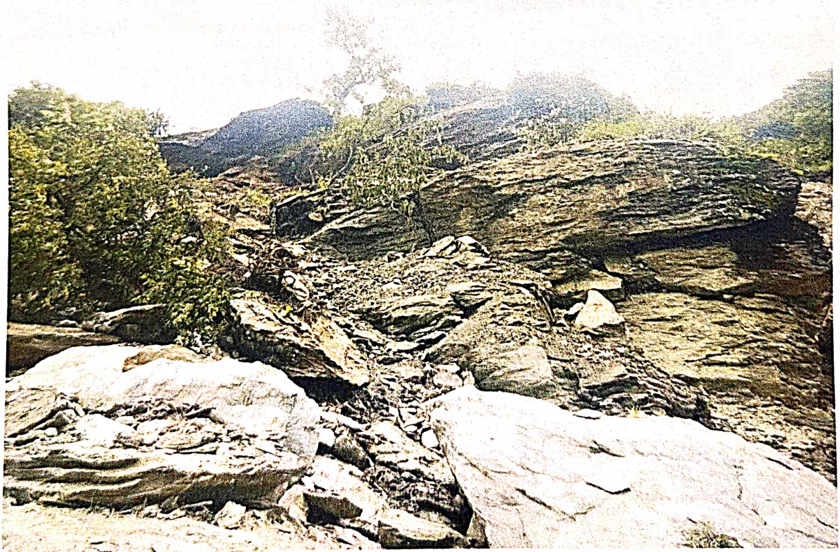
Slip and sliding Due to Monsoon
