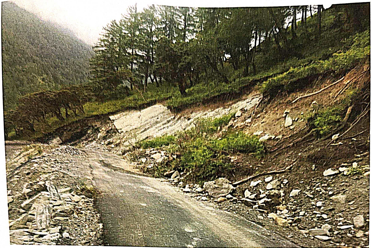
Slip and sliding Due to Monsoon
