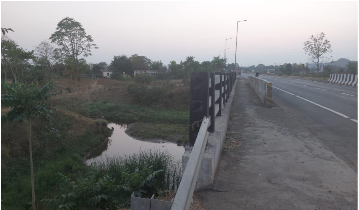
MNB at km 513.566
