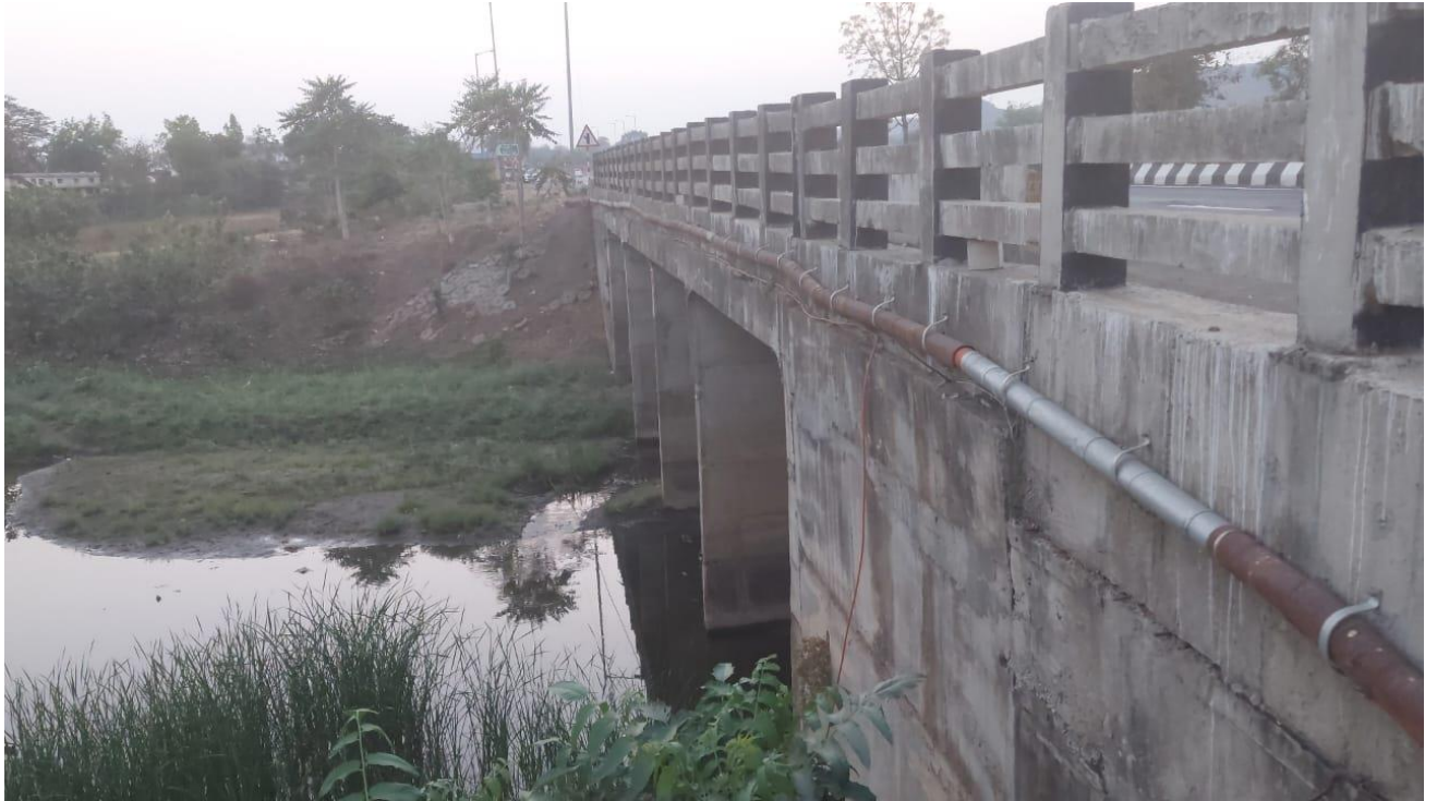
MNB at Km 509.760
