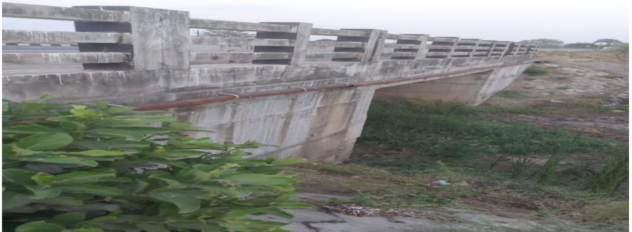
MNB at km 514.515
