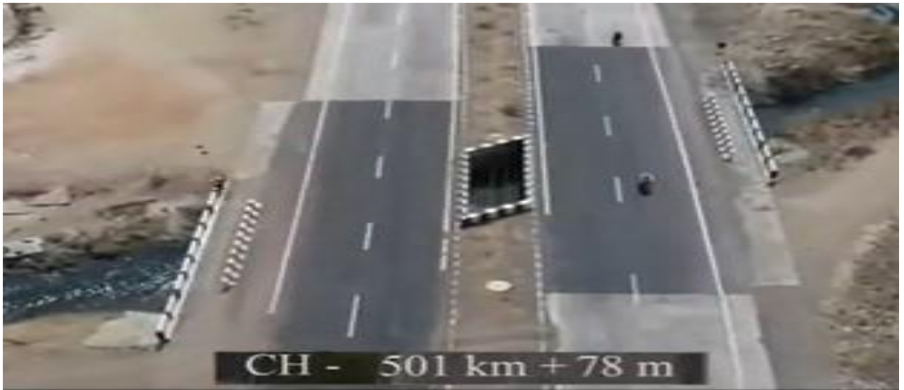
MNB at Km 501.103
