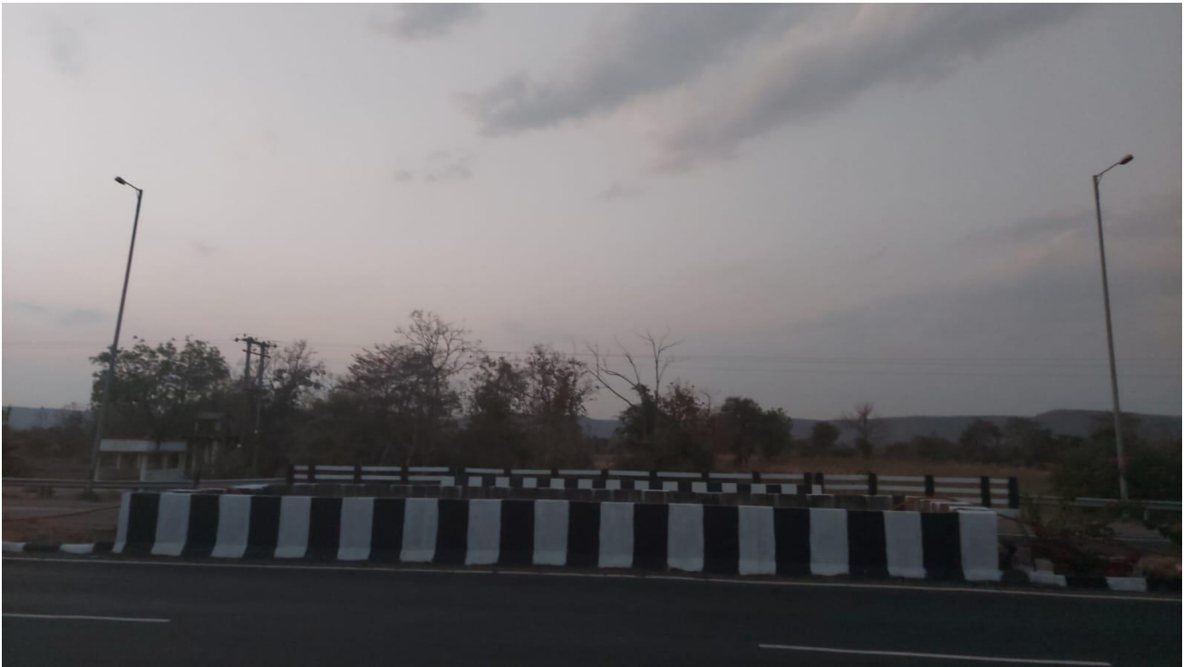
MNB at Km 508.583
