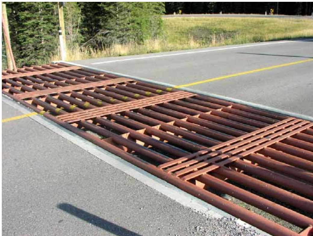
Figure 4. Cattle guards/grids to be installed at both ends of the crossing structure on NH 353 at Chainage 60/350 and 61/050. (Source: Clevenger & Huijser 2011)
