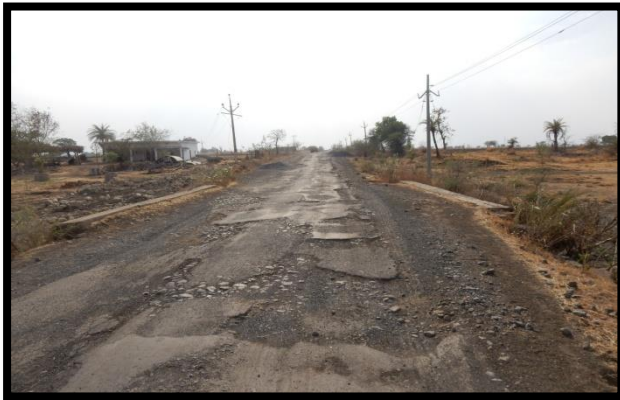
Figure 07:-Existing Pavement condition
