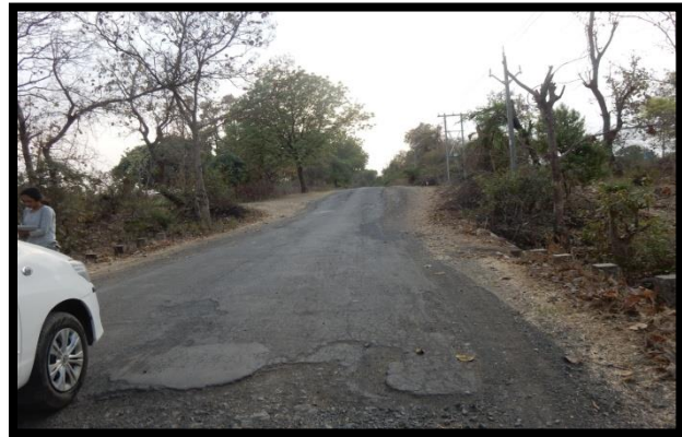
Figure 08:-Existing Pavement condition
