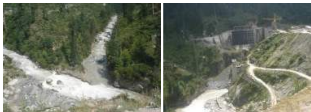
Tosh Nala and Parbati River Confluence Under construction dam of Parbati II HEP
