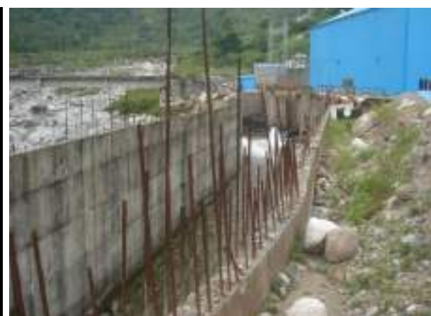
Power house site at Baner khad
