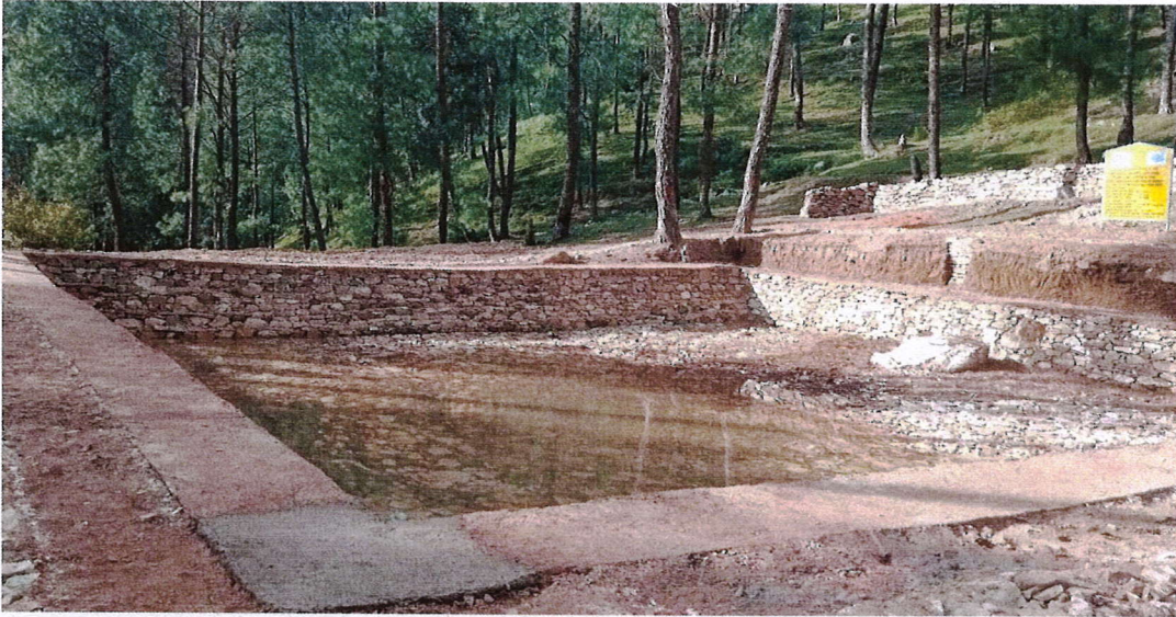
Water Harvesting Tank
