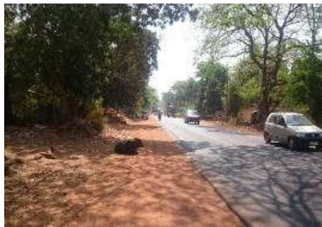
Rural area - Shoulder Condition @ Ch 179.200
