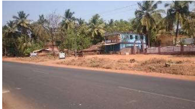
Pavement condition @ Ch 180.000
